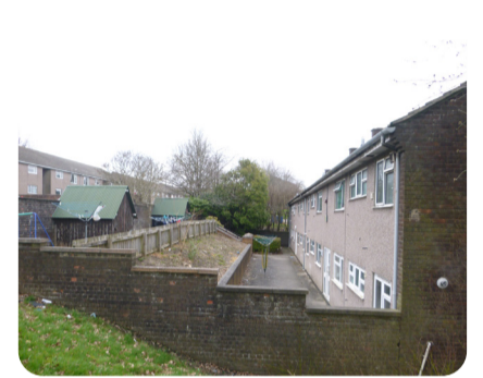
Showing steeply sloping gardens and retaining walls to the rears of the flats.
